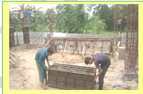
Picture-2 Construction worker without safety kits
