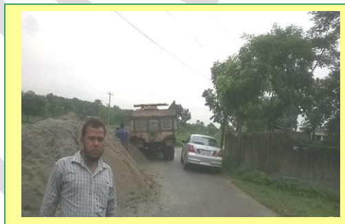
Picture-4 Construction materials dumped on the road side
